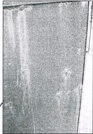
RUST ON PARAPET PANELS
