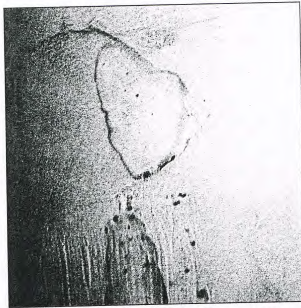
INTERIOR PLASTER WATER DAMAGE
