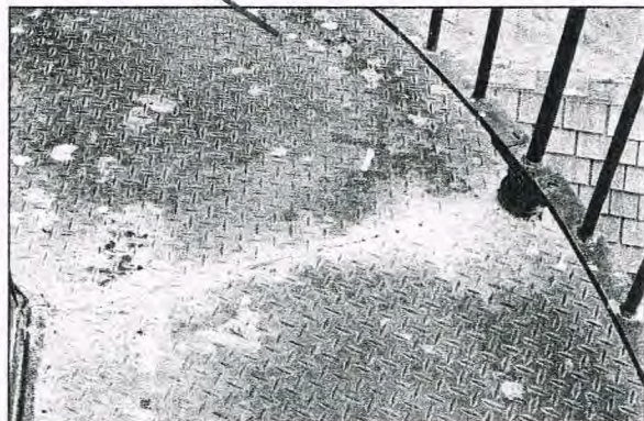
GALLERY DECK DETERIORATION
